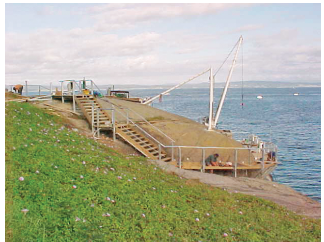
Figure 2. Construction of the walkway at Jetty Bay, Montague Island, that leads from the viewing platform (out of picture on left) to the wharf. Photo: Jack Babidge
